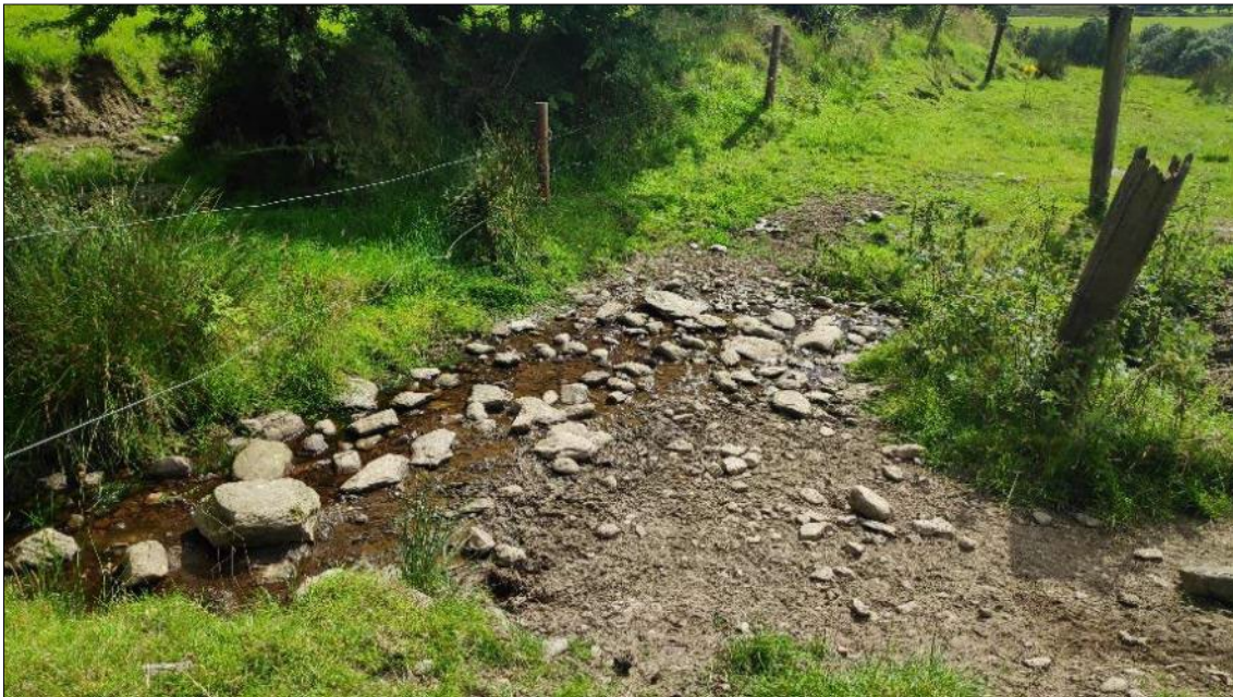
Plate 30: Representative image of site C14 the Clonavrick Stream (downstream of road culvert)
