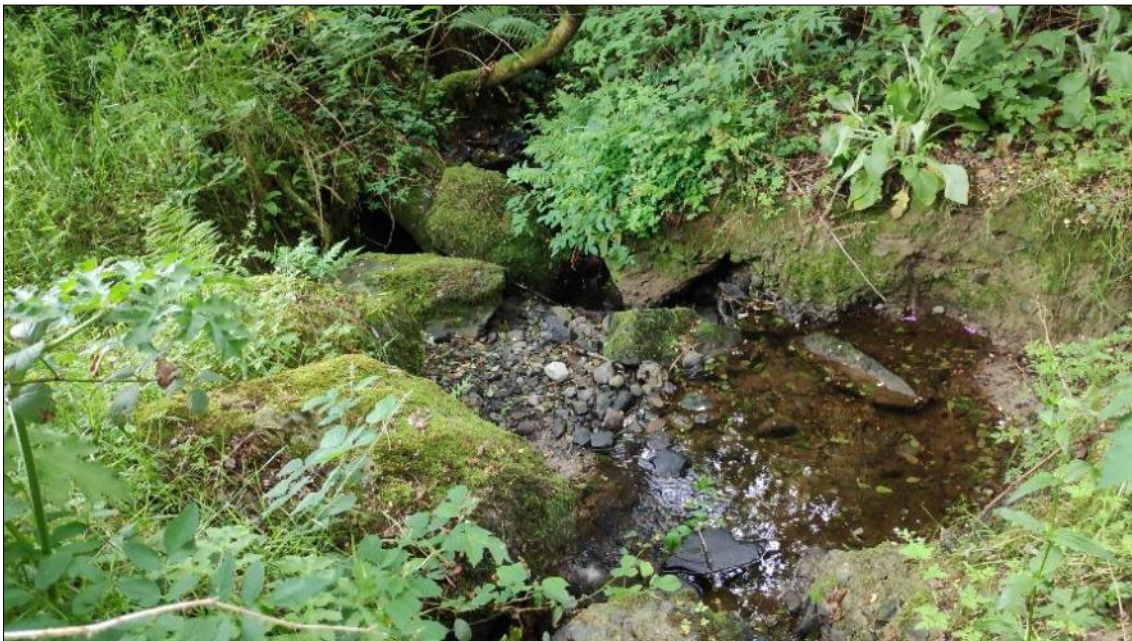
Plate 26: Representative image of site C10 on an unnamed stream at Carrigthomas, immediately downstream of the road culvert
