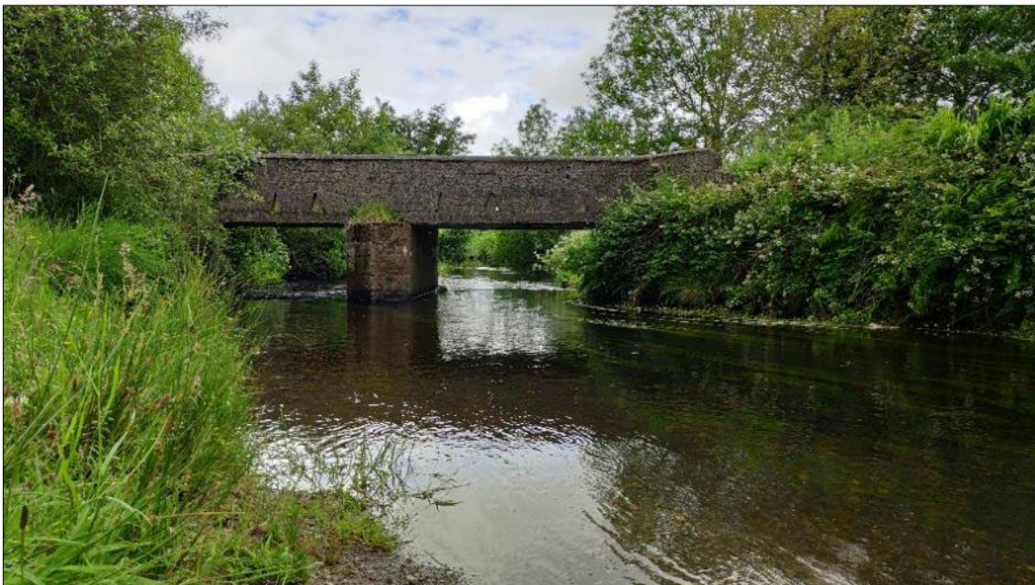
Plate 23: Representative image of site C7 on the River Laney at an unnamed bridge, Ballynagree West
